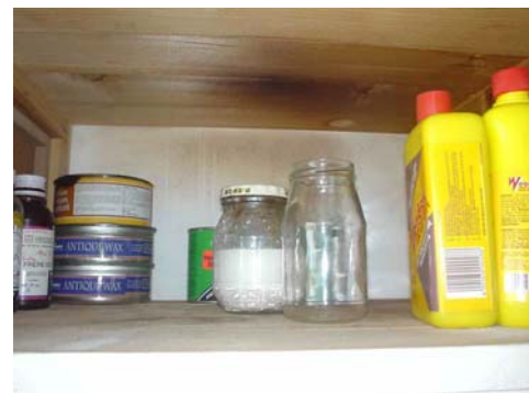
This is the shelf where the fire occurred. Note the singed underside of the next shelf.
